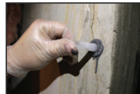
02: Press port firmly directly over crack
